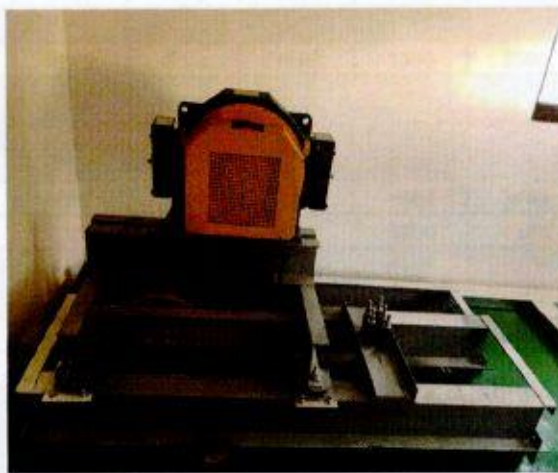
GEARLESS MACHINE MOUNTING ASSEMBLY IN THE MACHINE ROOM
